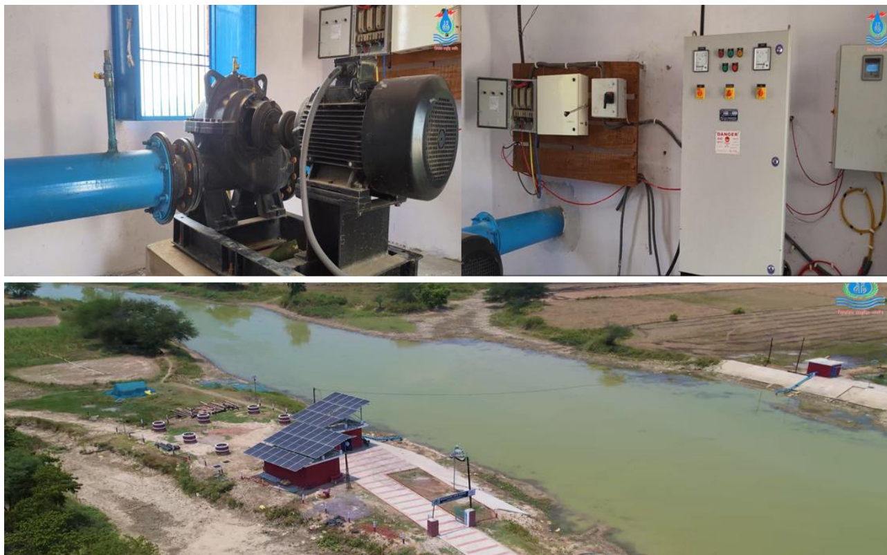
Figure 2. Integrated SPV-VFD Lift Irrigation System at Hriday Nagar: Pump-Motor Assembly, Electrical Control System, and Solar PV Installation at the Canal Site.
